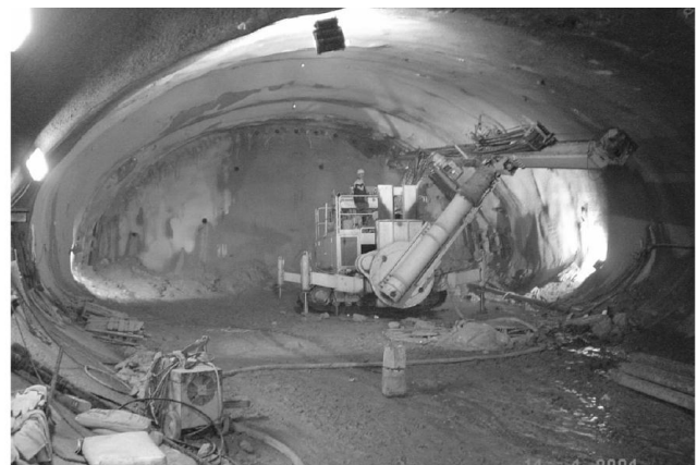
Figure 9: Installation of the forepoling tubes at the top heading of the station tunnel [7].
