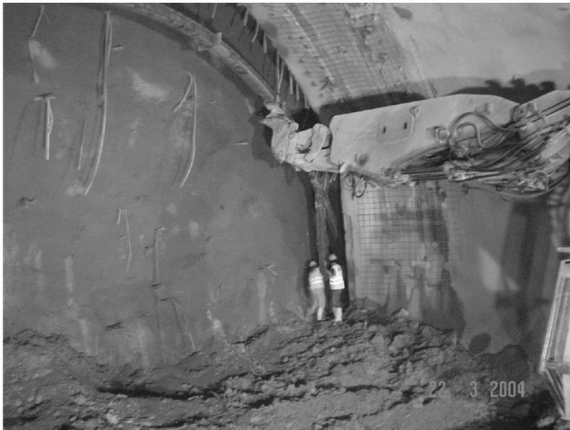
Figure 10: Top heading excavation of the station tunnel. Installation of the HEB 180 steel arches [7].
